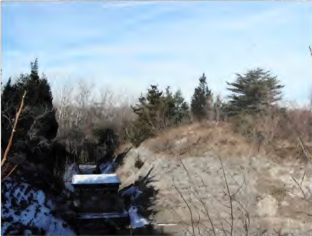
Figure 3.37. View looking west across southwest mortar pit, the Mortar Battery. Efflorescence and spalling are present on the concrete blast slope above the mortar pit. These symptoms of water infiltrating concrete can be seen on additional horizontal and vertical concrete surfaces at the Mortar Battery (Olmsted Center, January 2009).
